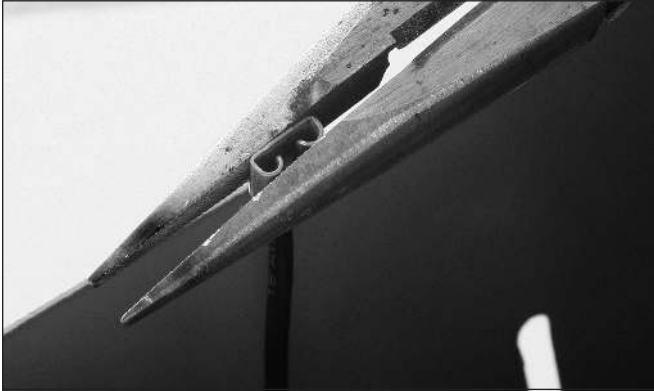
Squeeze loose push-on terminals with pliers to tighten. Replace terminals that show signs of heat damage.
