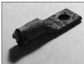
The wire burned off this terminal because of a loose connection.
