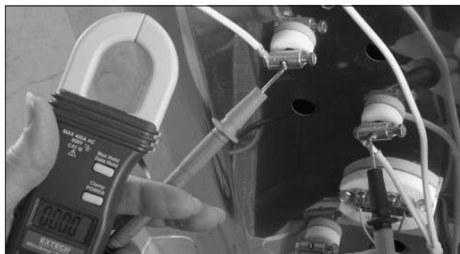
Testing an element with an ohmmeter. The ohmmeter leads are touching the two connectors of the element being tested.
