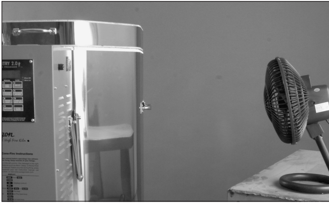
Lower the switch box temperature with air movement. This is especially useful during hot summers.
