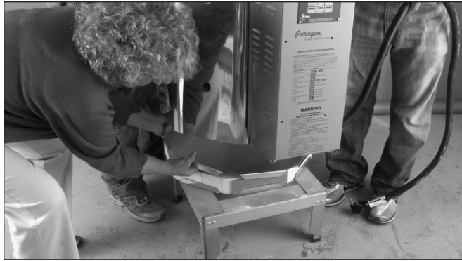
Place the new base plate on top of the brick bottom while your helpers hold up the kiln.
